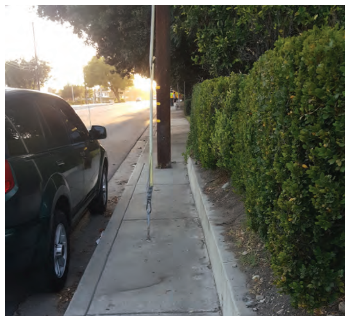
The greatest need for improved sidewalks on Arrow Highway is between Indian Hill Boulevard and College Avenue.
