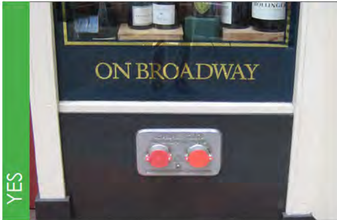
Example of an appropriately placed double standpipe connection in the base of a building at the sidewalk.
