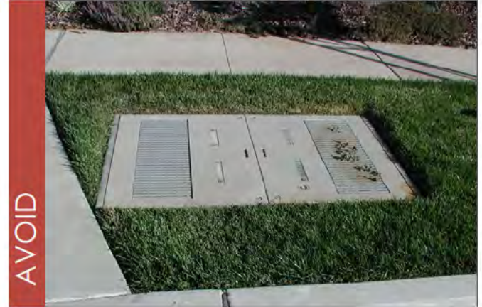
Example of inappropriately placed ground-level utilities in a parkway.
