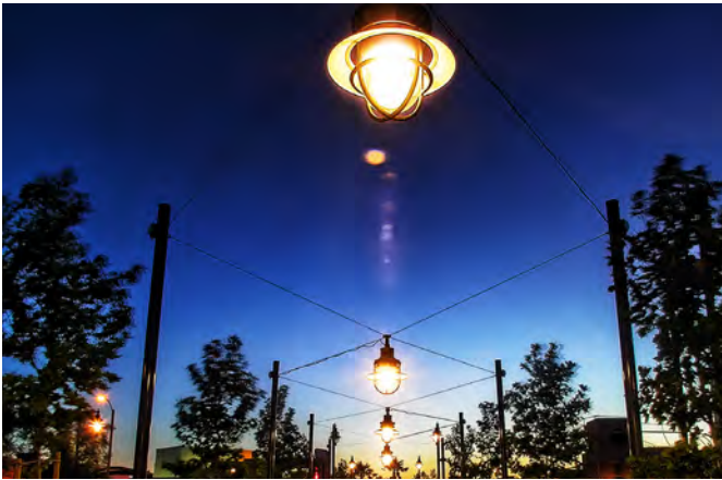
Suspended luminaires are aesthetically pleasing and interesting in parks and plazas.
