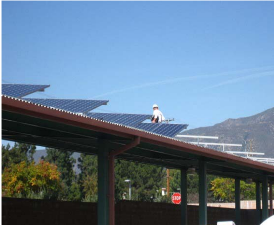
City Yard Solar Project
