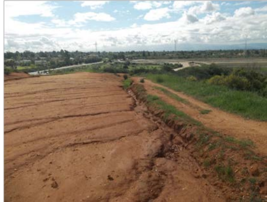
Extreme erosion on 5-mile Loop Trail Source: City of Claremont
